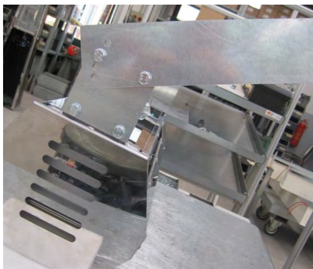
picture 1 – Installation at wall D-RAD
