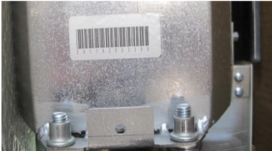
On the burner
